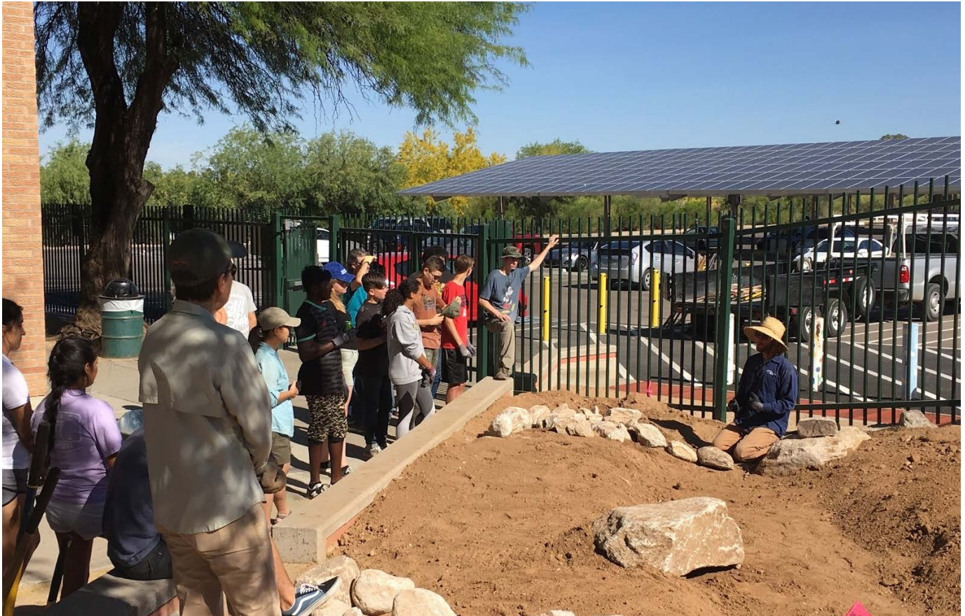
In May 2019, a group of volunteers gathered at Canyon del Oro High School in Arizona to install a rainwater garden. This is one example of eight similar projects at Tucson-area schools funded by NOAA's Environmental Literacy Program in which students developed rainwater garden plans with assistance from staff from Arizona Project WET and the Watershed Management Group. (Sarah Schoedinger, NOAA)
